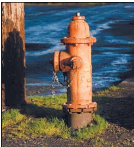
Benton County plans to add new fire hydrants in Alsea to help make the community safer in case of fire.
